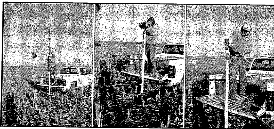
Figure 18. EnviroSMART probe installation. Photo on left shows auger being placed inside of the access tube. Center photo shows auguring of the pilot hole and the photo on the far right shows the access tube being pounded into the ground after auguring. This process was repeated several times to complete the access tube installation.
