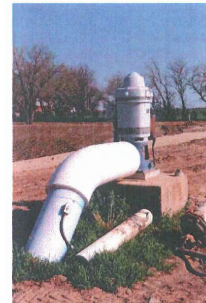
Example of Recovery Well
