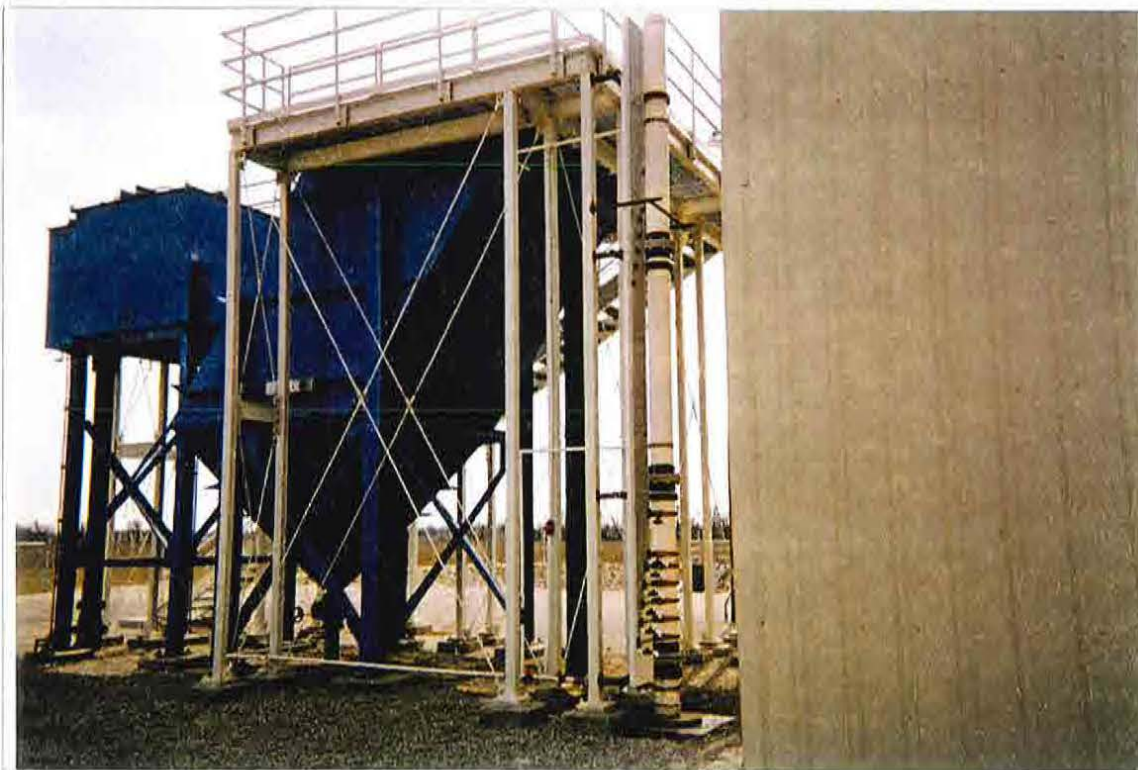
Filter Column Adjacent to Treatment Facilities - Sedgwick Intake Site May 24, 1999
