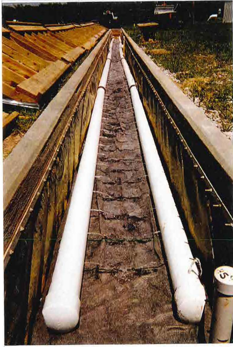
Distribution Piping Halstead Recharge Site May 1999
