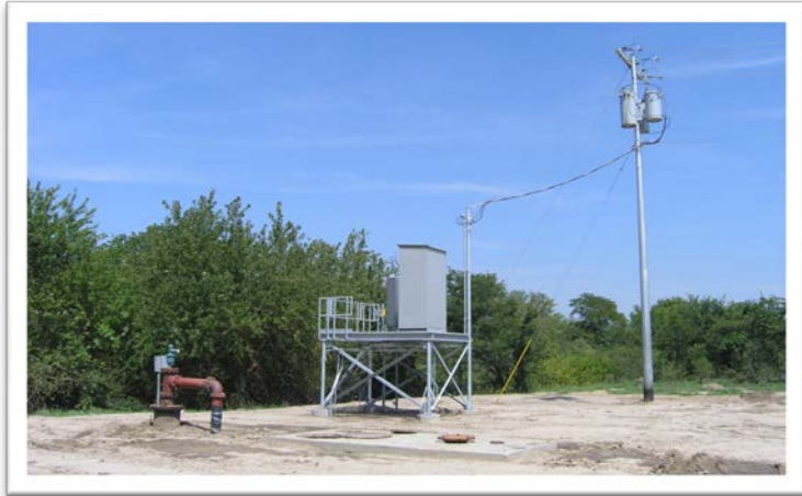
Bank Storage Wells
