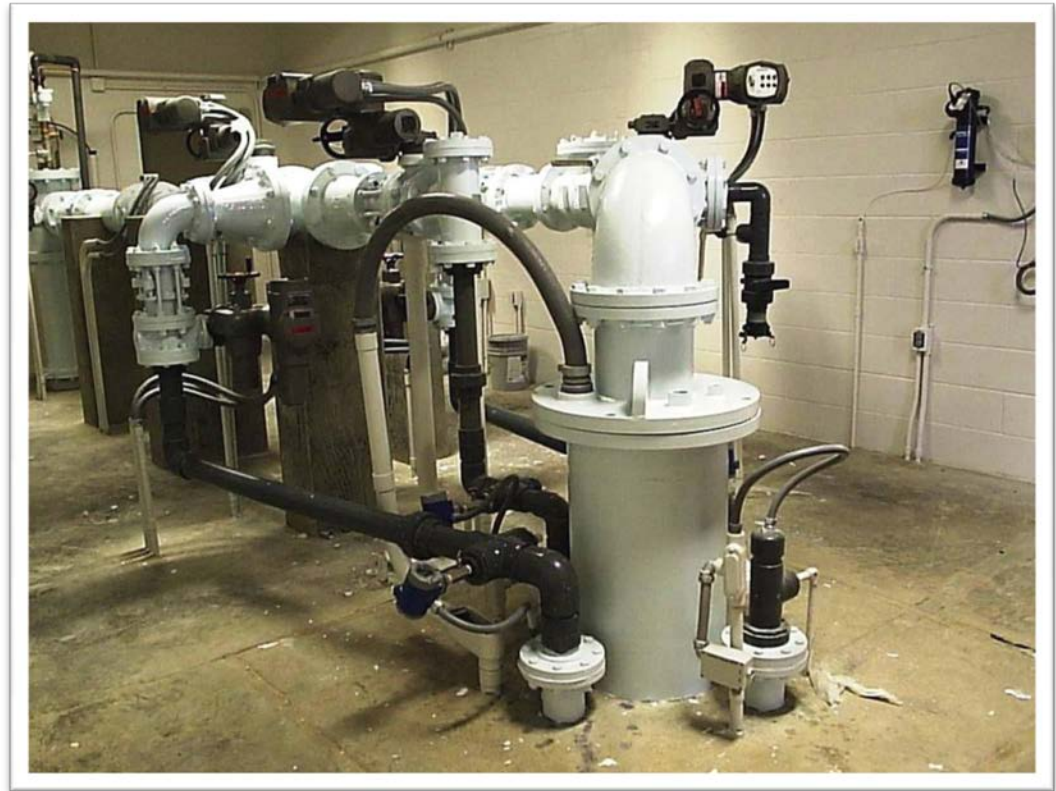
Recharge Recovery Wells (RRWs)
